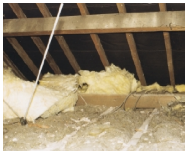
Figure 5 This photograph from the local authority study shows the additional layer of mineral fibre insulation missing from a substantial portion of the loft.
