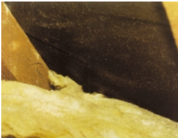
Image 2 This image is of property #57 Street A. It shows mineral fibre blocking eaves ventilation.
