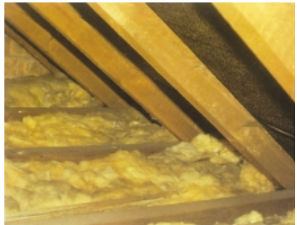
Image 3 This image is of property #4 Street B. It shows mineral fibre blocking eaves ventilation.
