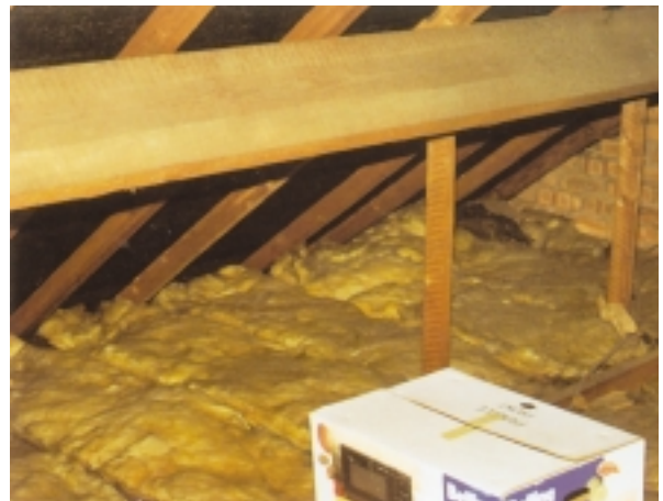
Image 4 This image is of property #36 Street B. It shows mineral fibre blocking eaves ventilation.
