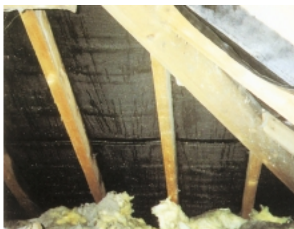
Images 8 & 9 These images are of properties #51 & 57 Street A. They show condensation occurring on the underside of the sarking felt with a greater concentration of droplets around the lower levels of the roof space.
