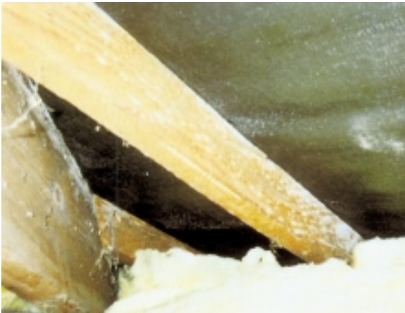
Images 10, 11 & 12 These images are of properties #81 & 83 Street A. They show signs of mould growth on rafter sides.
